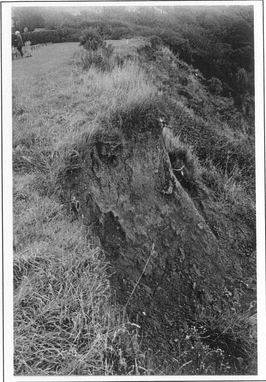
Plate 7 – High angled debris slide on north westerly facing slope showing drainage pipe.
